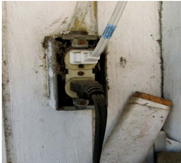
Figure 25: Dangerous Electrical Outlets Are a Common Problem in Puerto Rico
