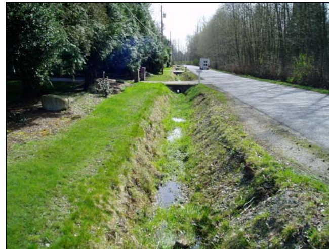
Photograph 20 – Downstream view of 164 th Street East ditch. Increased flow with localized scour, mineral alluvium and direct connectivity to Class A watercourse below 16 th Avenue.
