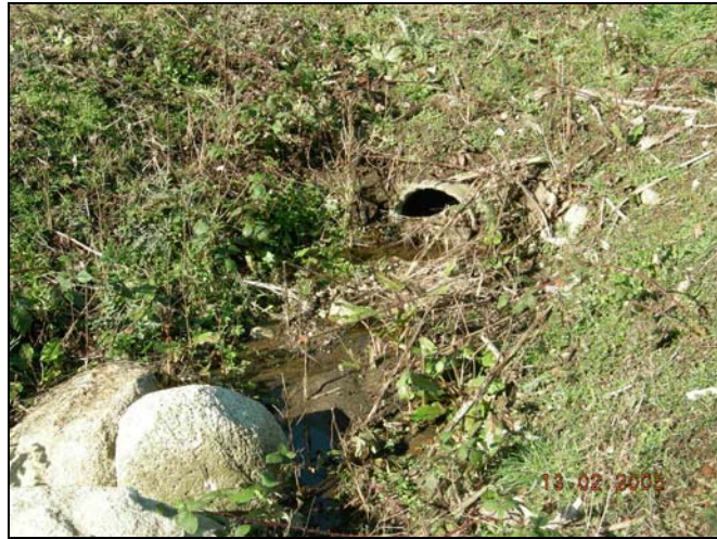
Photograph 22 – Manmade drainage ditch located north of residential property at 16691 16 th Avenue. No direct downstream connectivity.
