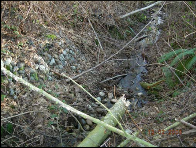
Photograph 17 – Downstream view of 164 th Street right-of-way channel. Rock gabion weirs located throughout channel length.
