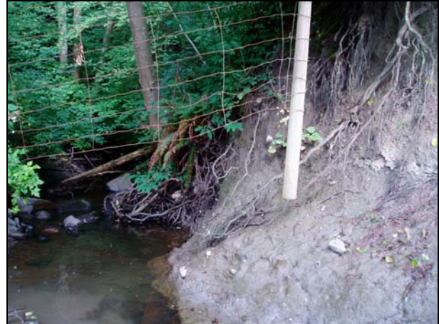
Photograph 8 – Downstream view of bank erosion/channel widening below Highway 99 culvert outlet. Note hanging fence post depicting the relatively recent changes to the channel.
