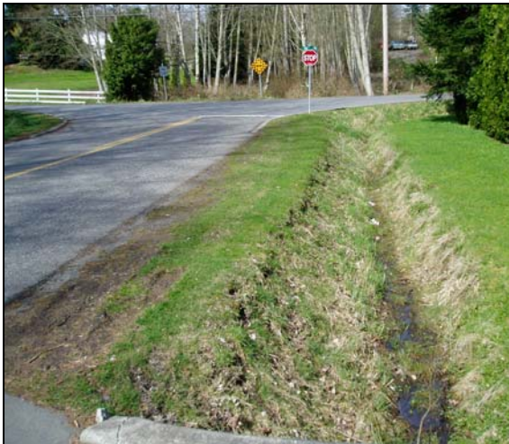
Photograph 19 – 164 th Street East ditch below 20 th Avenue. Grass lined ditch with negligible flow and no significant scour.
