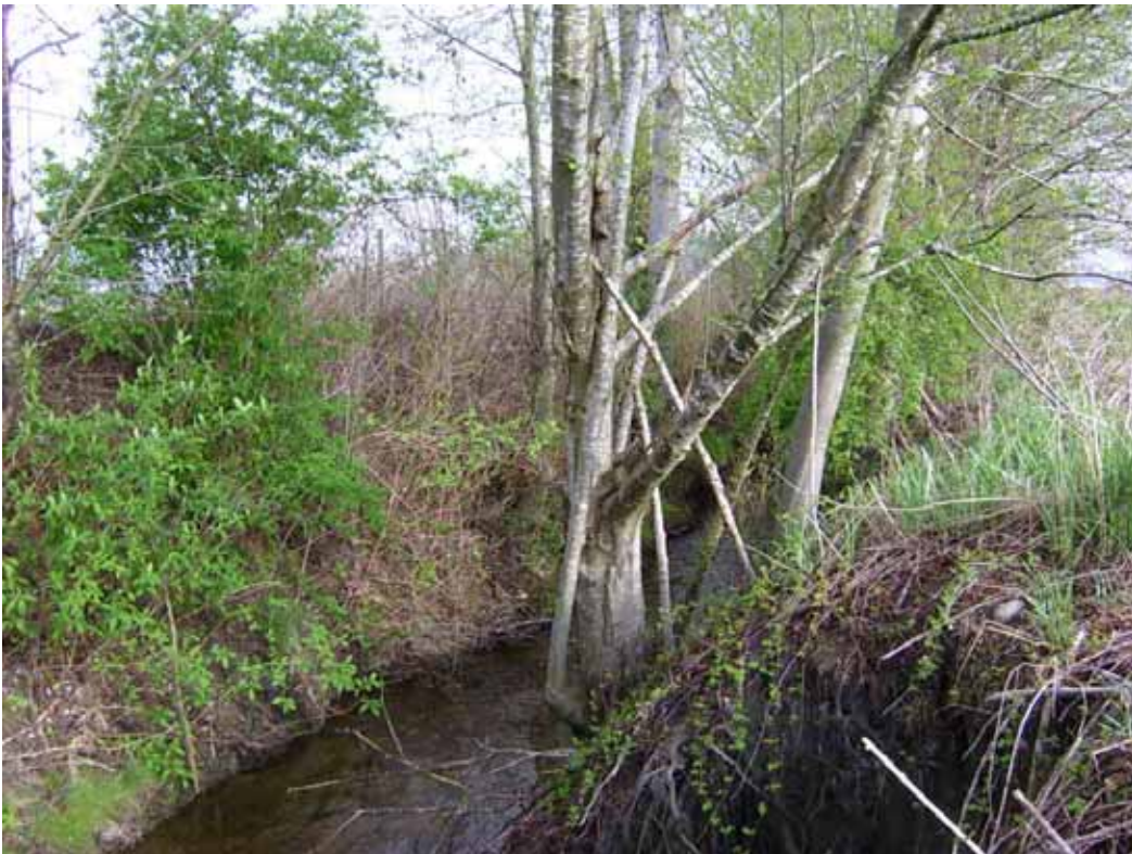
Photo 46: 180 th Street ditch shows signs of erosion.
