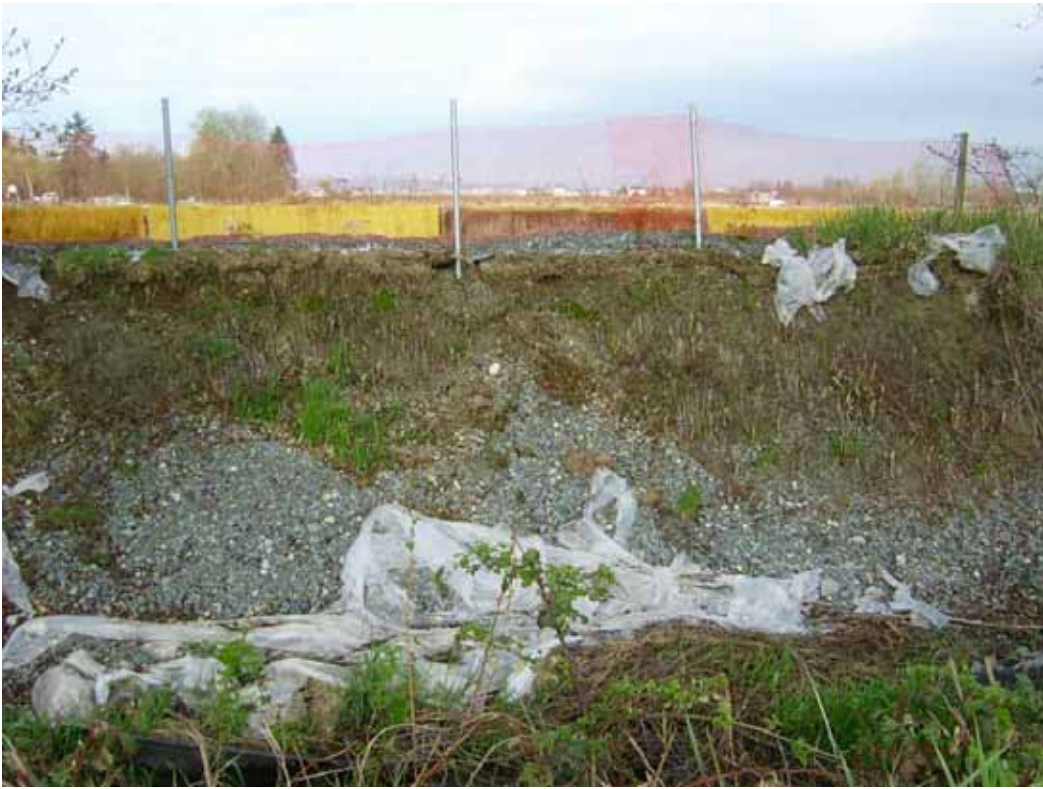
Photo 47: 180 th Street ditch shows signs of erosion.
