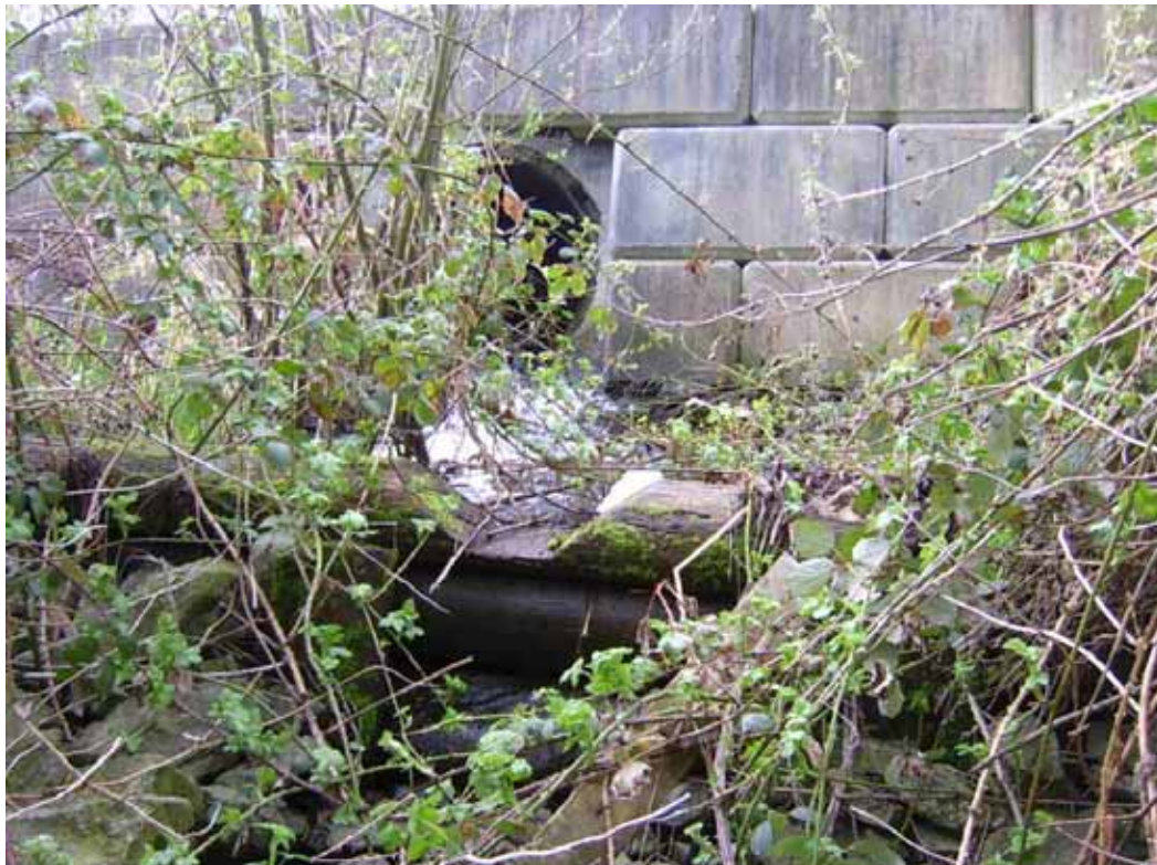
Photo 7: EC-3 presents a possible barrier to fish migration. Water flows around the wooden weir when flows are low and may make passage difficult for fish.
