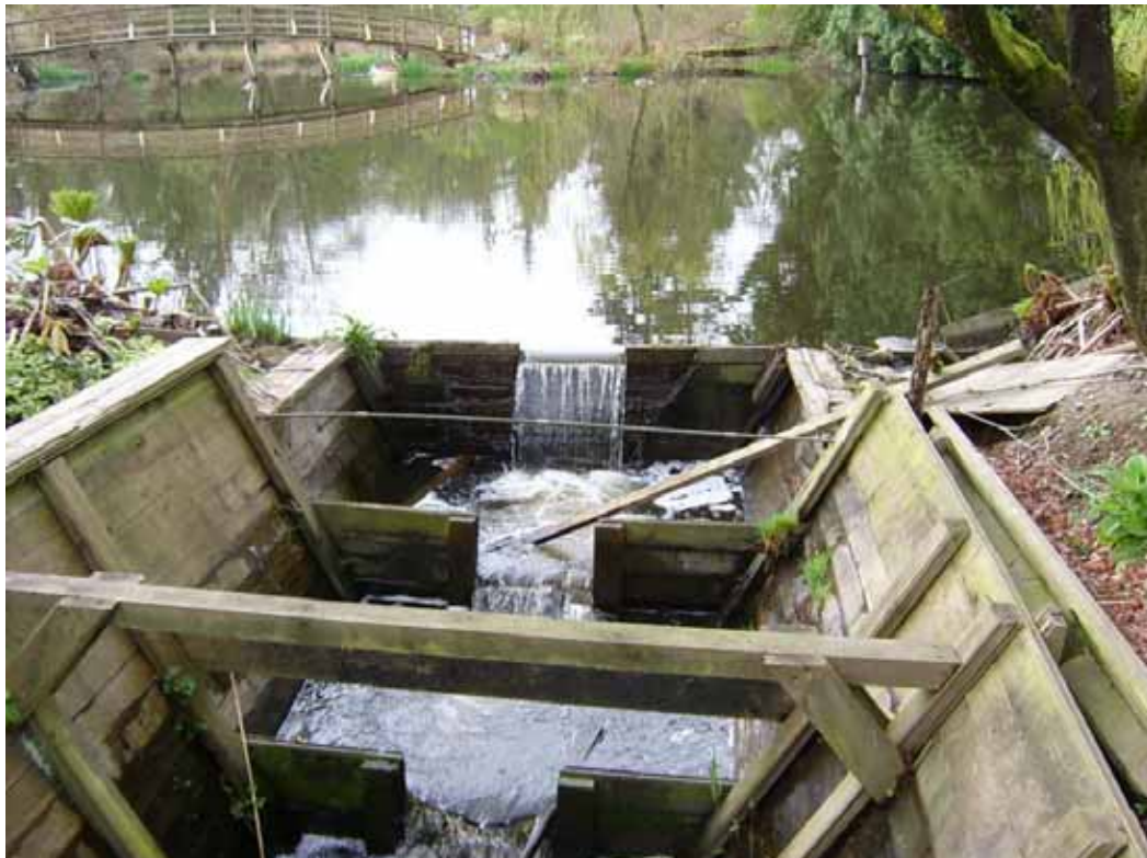
Photo 9: Fish ladder at EC-4, directly south of 29A Avenue.
