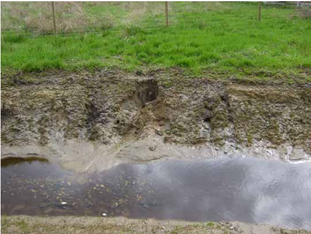
Photo 44: 184 th Street ditch shows signs of erosion.
