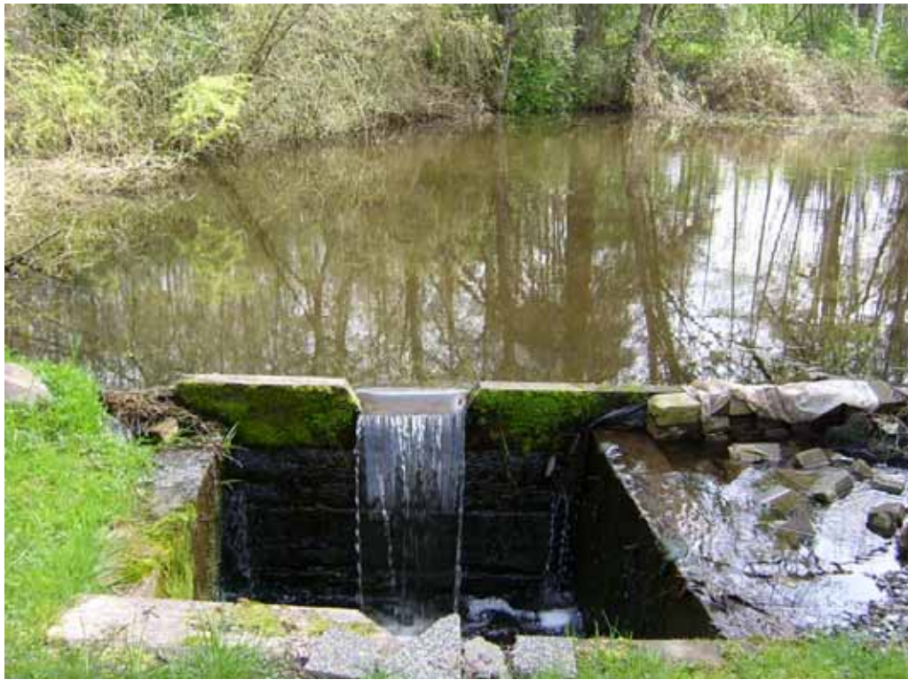
Photo 11: Pond outlet in EC-4 may present a barrier during low flow (0.94 m drop measured during April assessment).
