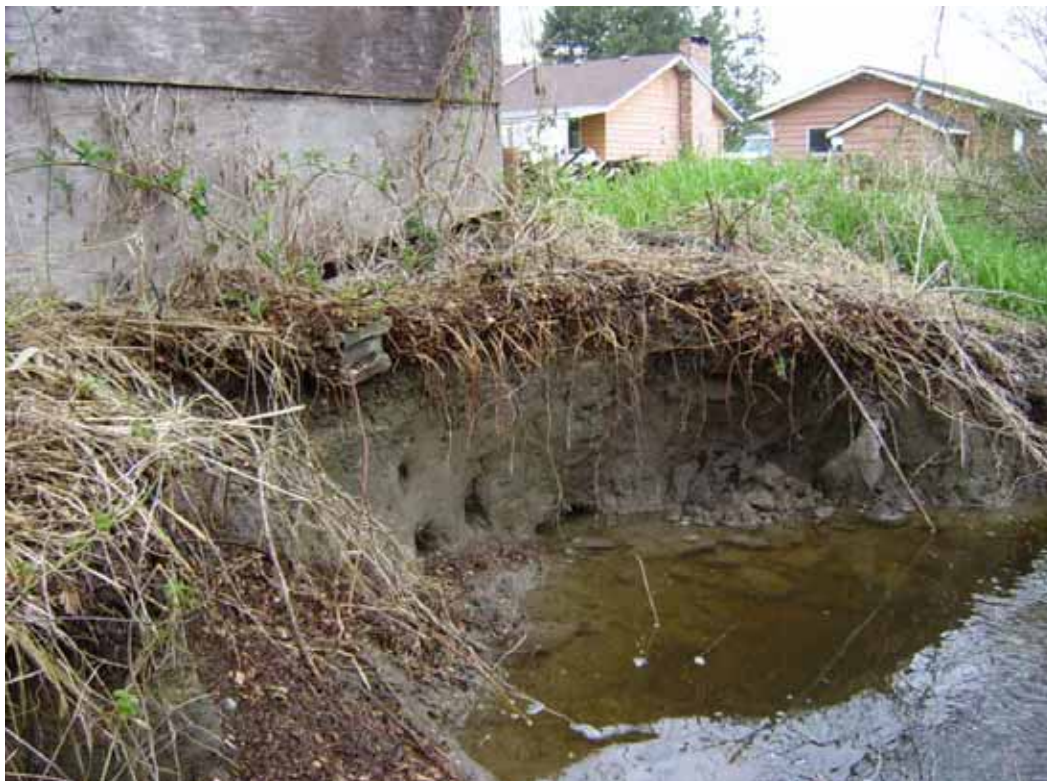
Photo 4: Some bank erosion at EC-1.
