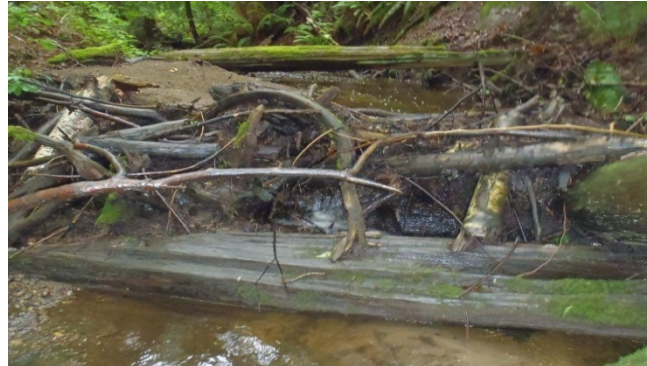
Photo D Debris Jam and Sediment Wedge
