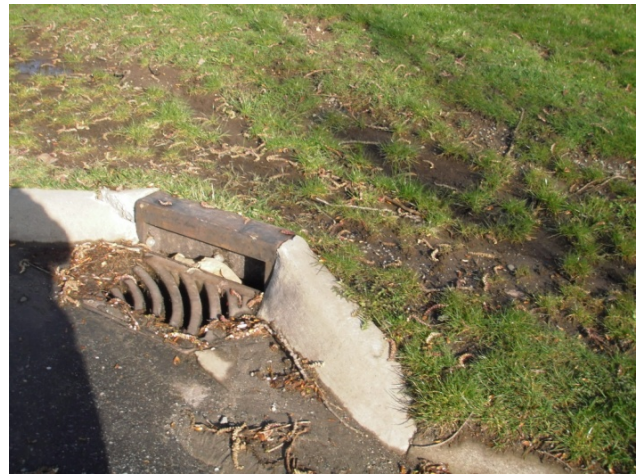
Figure A.14: Swale Separated from Roadside Catch Basin by Curb.
