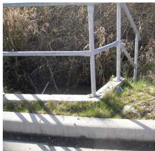
Figure A.3: Overgrown ditch outlet for storm sewer system
