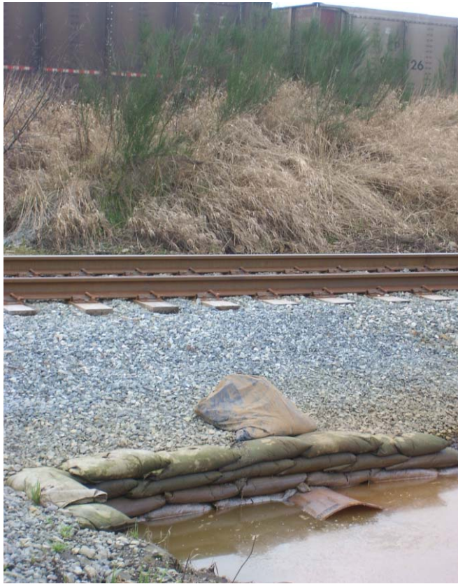
Photo 5: Culvert across the Railway along 176 St. (view from south side of the rail)
