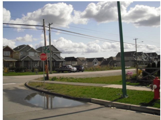
Figure A.16: ponding against curb
