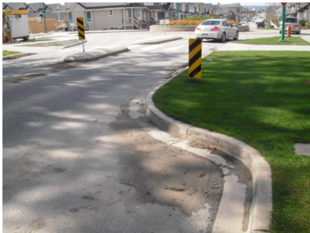
Figure A.15: Sediment buildup along curb
