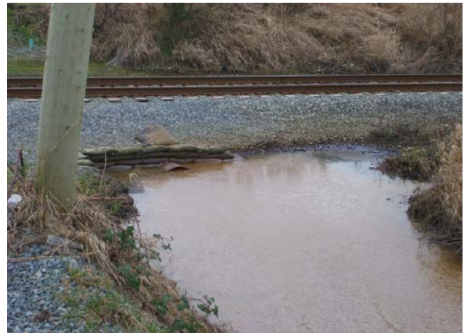
Photo 4: Culvert across the Railway along 176 St. (view from north side of the rail)
