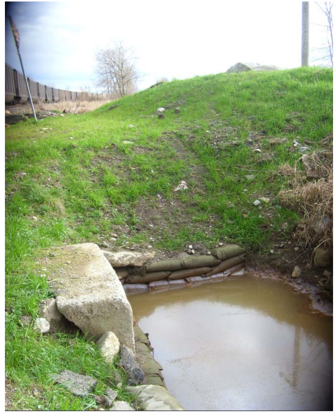
Photo 6: Drainage system along the Railway corner of 176 St. and Colebrook Rd (view from south side of the rail)
