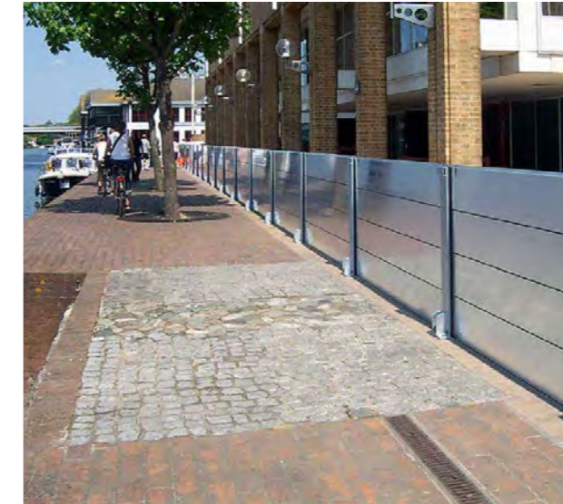
Removeable flood barriers
