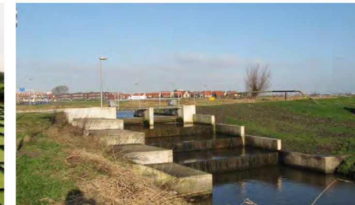
Pumping station Meerpolder, NL
