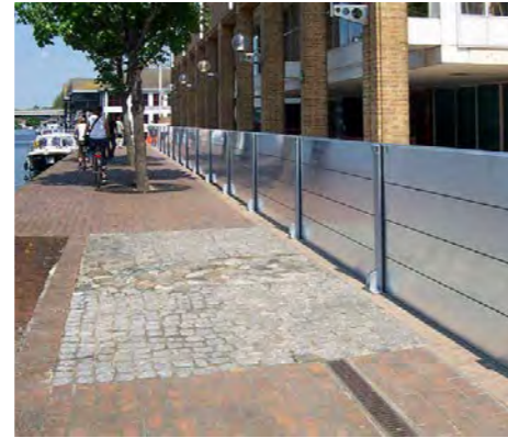
Removeable flood barriers
