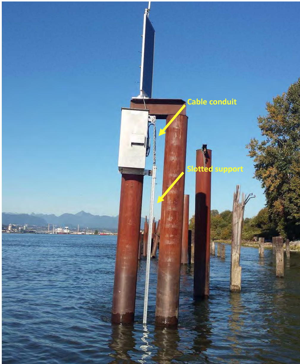
Figure 1 Example of a combined cable conduit and slotted support mounted to a pile. A similar configuration will be used at the Crescent Channel Nearshore Wind and Wave Monitoring Station; however the slotted support will be larger diameter.
