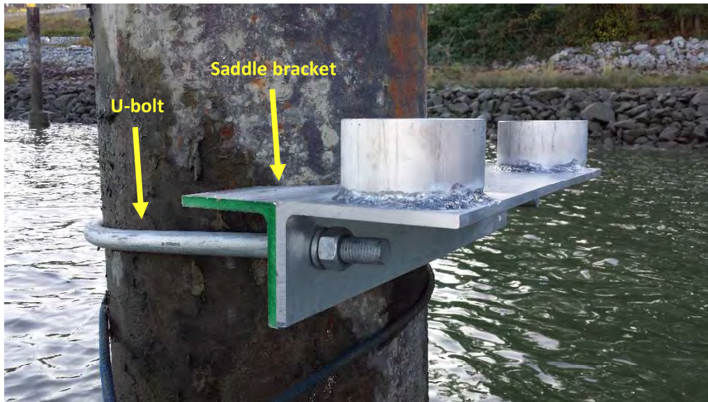
Figure 2 Example of a U-bolt and saddle bracket around a pile. A similar configuration will be used to affix the slotted support track at the Crescent Channel Nearshore Wind and Wave Monitoring Station above the installation water level.
