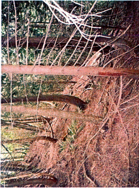
PHOTO 13 – Curved Trees Indicating Slope Movement
