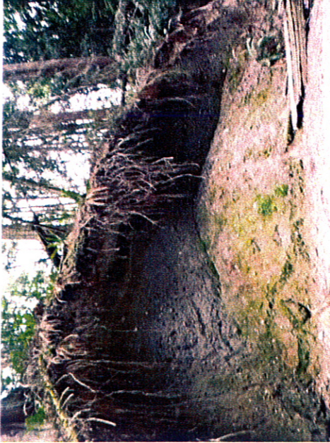
Photo 1 – Erosion Resulting in Overhang
