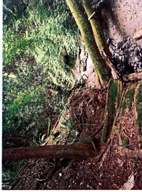
PHOTO 8 – Fallen Undermined Trees
