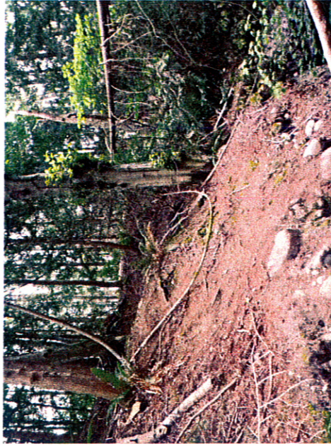
PHOTO 7 – Soughing Slope with Associated Leaning/ Curved Trees
