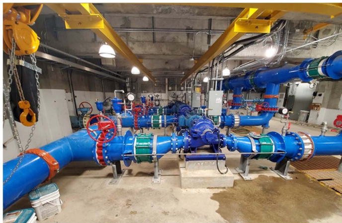
Drinking Water Pump Station
