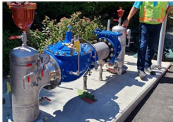
New Above Ground PRV Station
