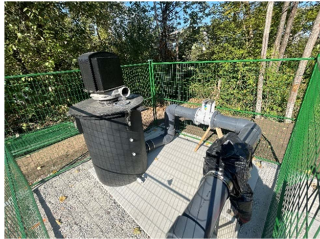
Odour control unit on Roxburgh Road
