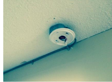
Disabled Hard Wired Smoke Alarm
