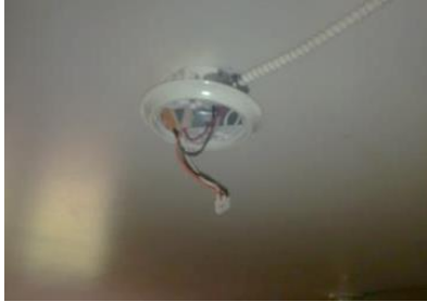
Disconnected Smoke Alarm
